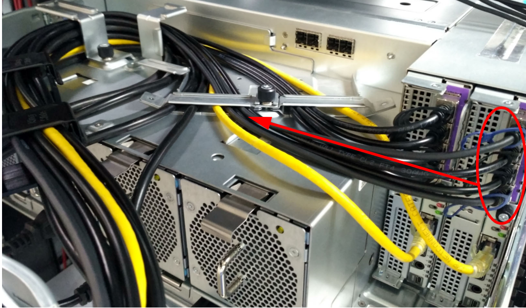
Figure 58 Routing 10GbE SFP+ cables of the right controller
