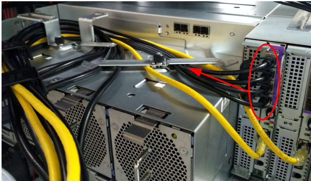
Figure 57 Routing 10GbE SFP+ cables of the left controller
